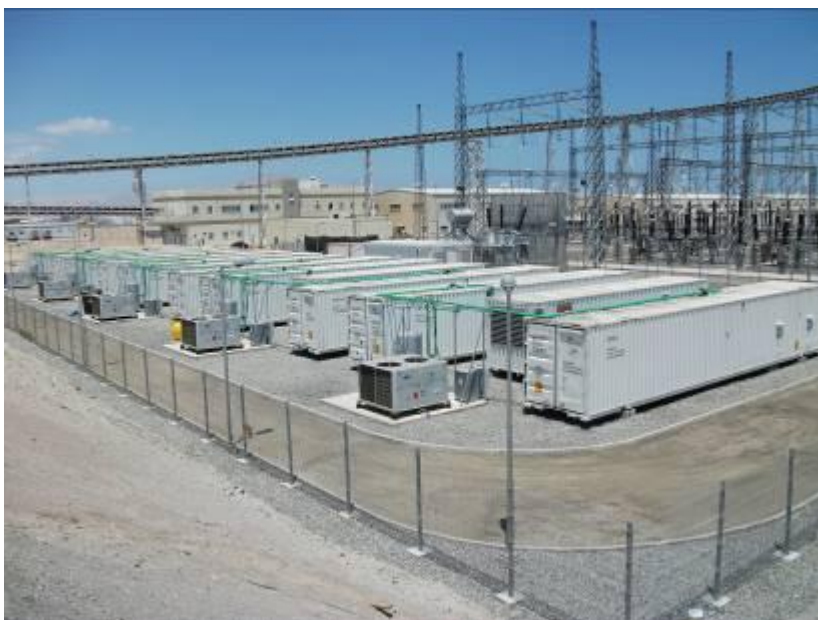
Figura 2.12 BESS de litio, Los Andes AesGener [7]
