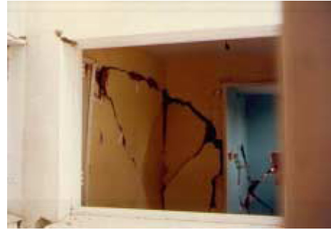
(b) Crack pattern in the masonry panel.
