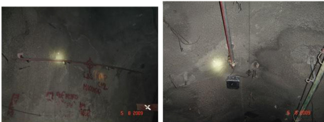
Fig. 10. Tube sensors attached to tunnel sidewall and ceiling.
