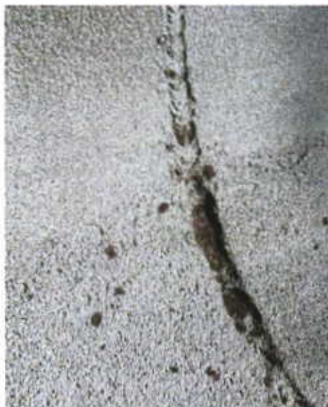
Figure 16b: Localized metal loss feature in girth weld
