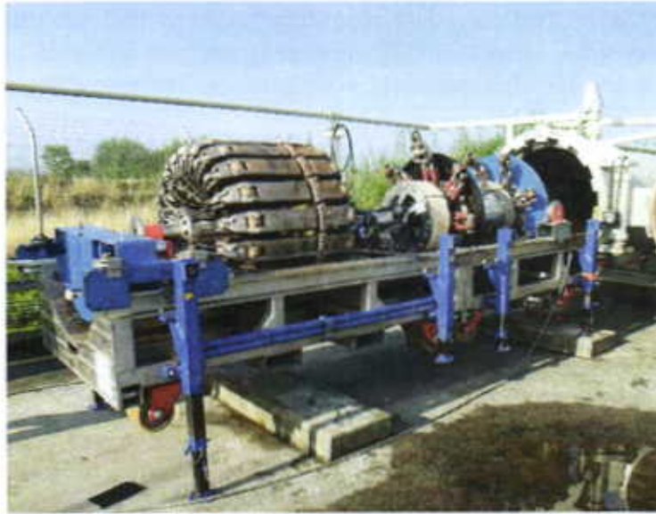
Figure 11: Launch of multi-technology tool in a 42" gas pipeline
