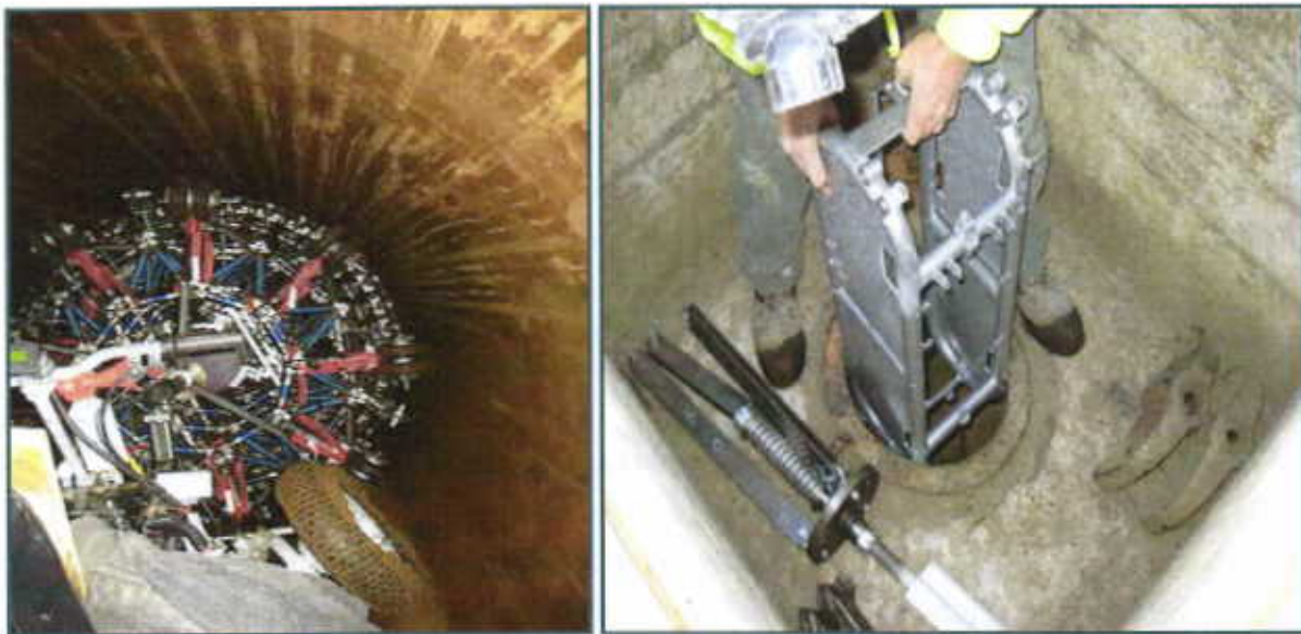
The view of the MFL tool from the propulsion vehicle driver's seat, and assembly of the vehicle from parts handed through an access manway in the pipeline.
