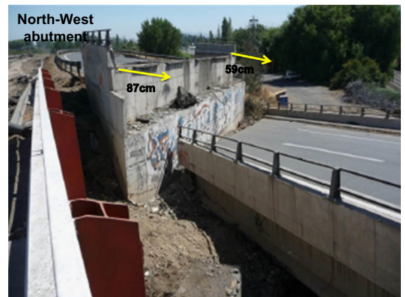
Fig. 26. Collapse of Hospital overpass.
