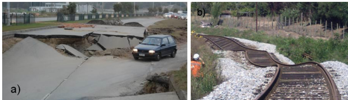
Fig. 14. Post-liquefaction settlements. (a) Costanera route in Concepción and (b) near Concepción City (EFE).
