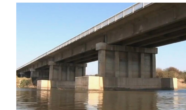
Fig. 24. (a) Plan and elevation of original piers (modified from [26]) and (b) Repaired piers after 1985 Earthquake (Videos MOP).
