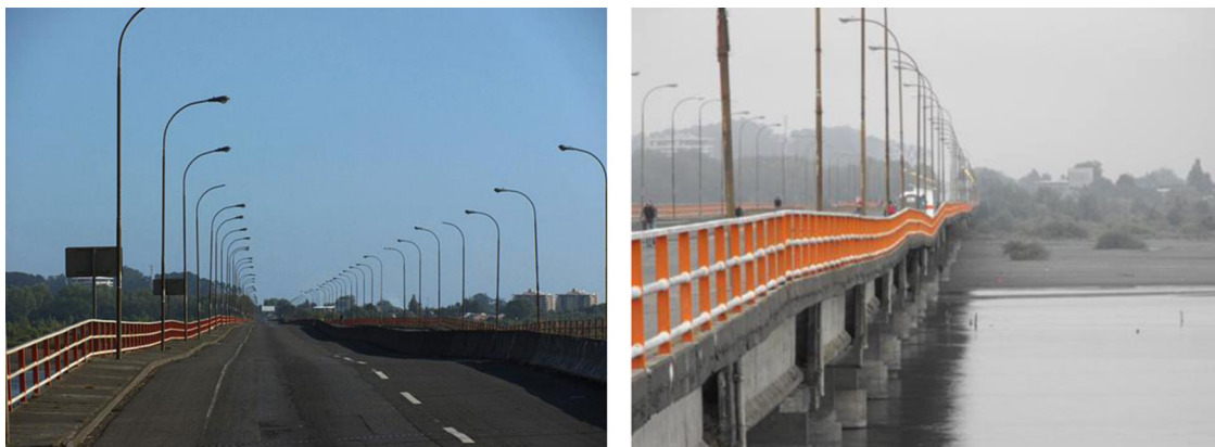
Fig. 20. Settlements along Juan Pablo II Bridge with no evidence of horizontal displacements.
