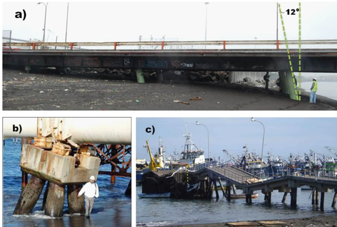
Fig. 18. Lateral spreading, (a) Coronel Port, (b) Bocamina Port and (c) Fishermen's Port.
