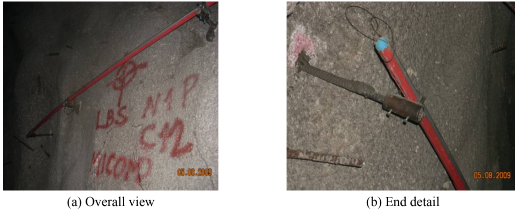
Fig. 6 Sensor tubes attached to the tunnel sidewall
