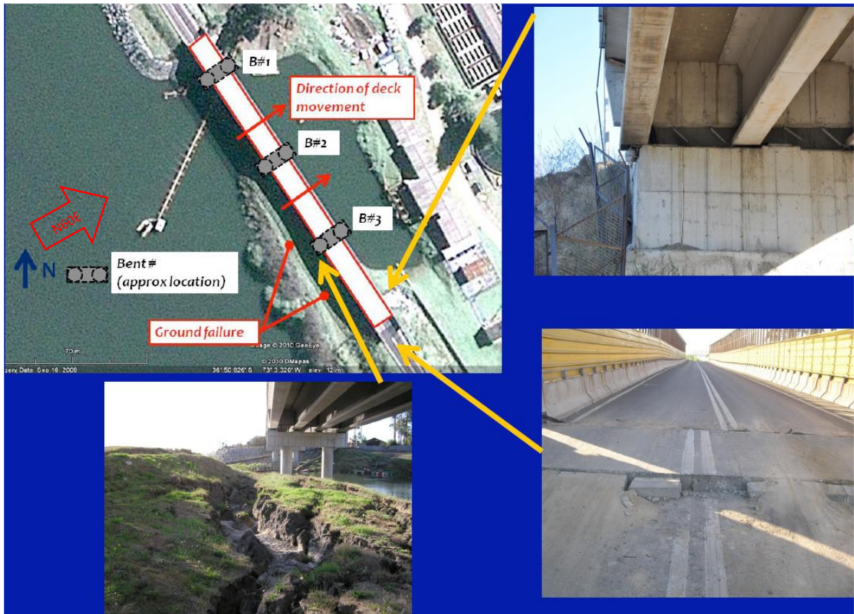
Fig. 5.45 Daños en puente La Mochita (Imagen Geo-engineering Reconnaissance of the 2010 Maule, Chile Earthquake).
