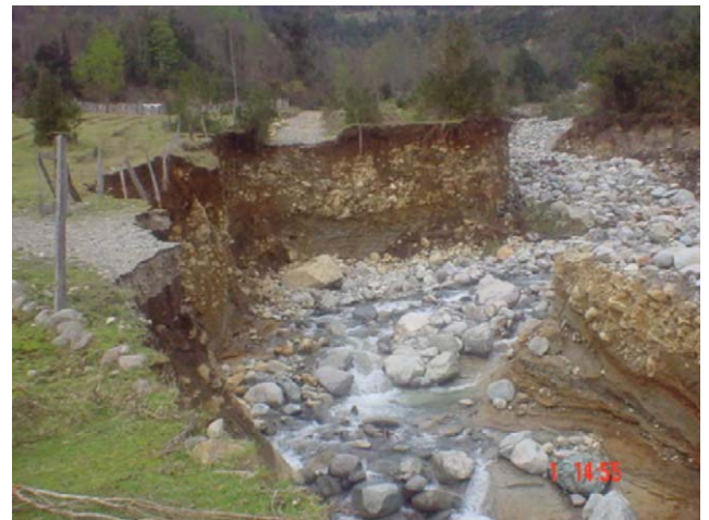
Fig. 10. Gully formed by the Coquimbo Creek debris flow in Lake Ranco, due to erosion of Holocene landslide and alluvial deposits. Note the dirt roads cut by the gully.
