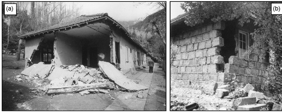
Fig. 4. Damage in unreinforced masonry house in El Volcán (a) and Las Melosas (b) (DIC, 1958) after the event on 4 September 1958; see location in Fig. 2.
