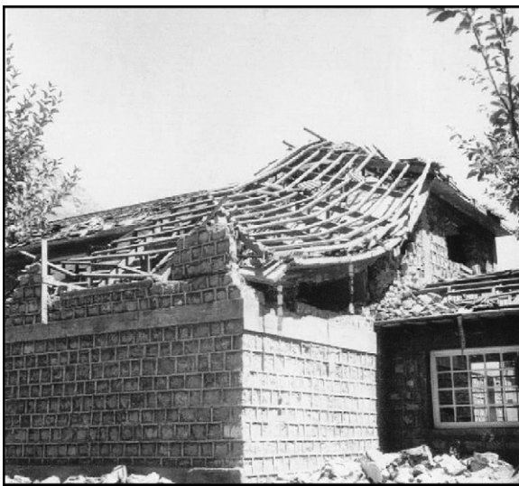
Fig. 5. Damage in two story unreinforced stone masonry buildings in Las Melosas after the earthquake on 4 September 1958 (DIC, 1958); see location in Fig. 2.
