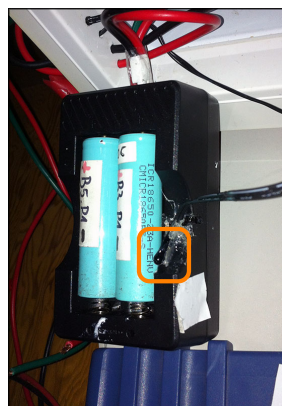
Figure 3.3: Photography of the battery case, showing with an orange circle the location of the sensor near to the negative pole.
