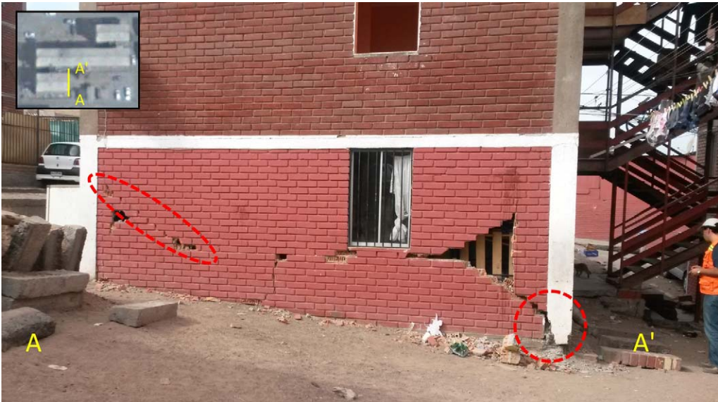
Figure 10. Observed damage in buildings type A in Dunas I.
