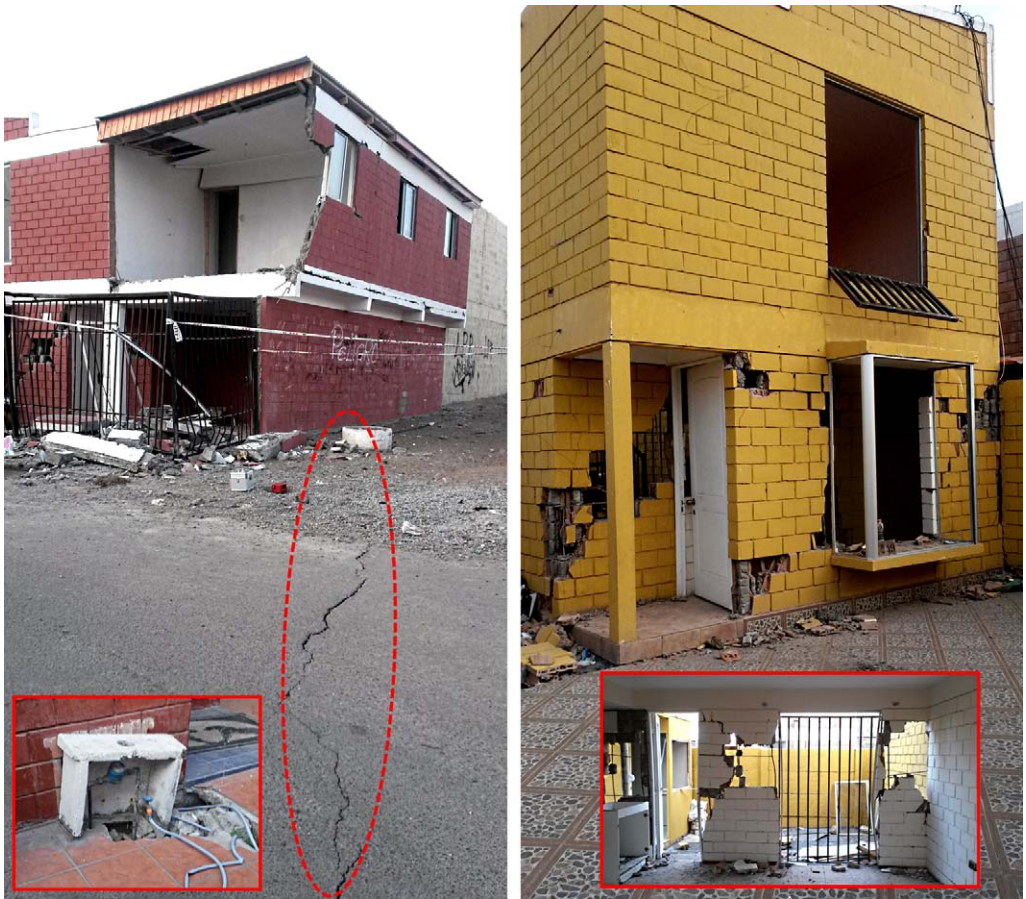
Figure 13. Observed damage for Houses 1 and 2. (a) House 1 shows post-seismic cracks and identified cavities, and (b) House 2 illustrates the most damaged house in Santa Eloisa condominium.
