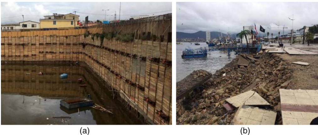
Figure 7. (a) Flooded excavation in Coquimbo (29.958°S, 71.338°W). No damage observed on the soldier piles and anchors; (b) failure of gravity walls at Coquimbo's waterfront (29.951°S, 71.336°W).
