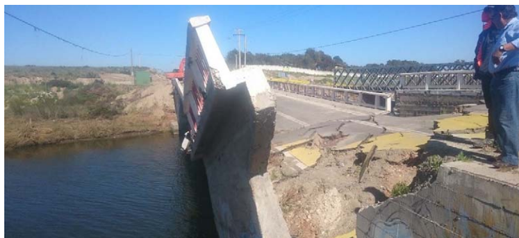
Figure 11. Field photograph looking south of the D-420 bridge. Northern end of the bridge has a vertical step where it failed during the earthquake. People shown for scale (30.261°S, 71.481°W).
