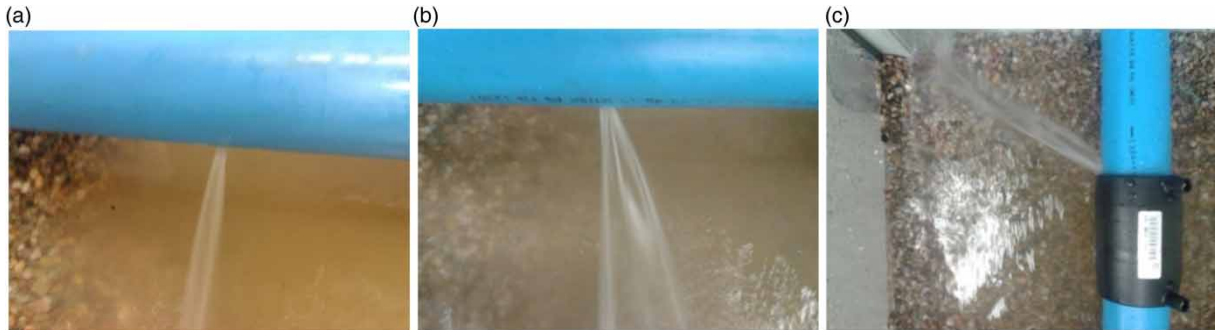
Figure 3 | Photographs of leaks: (a) round hole; (b) longitudinal slit; (c) electrofusion joint.
