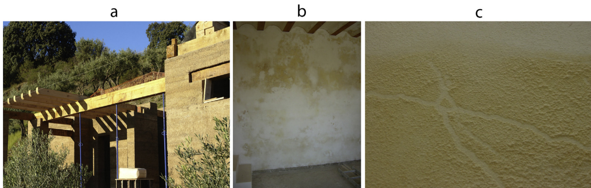
Fig. 1. (a) A house built with rammed hemp concrete walls; (b) pathologies arisen on the plaster of a hemp concrete wall on the inner Northern side of a hemp concrete building (c) detail of the powdered aspect of the yellowish deposition on the same plaster. (For interpretation of the references to colour in this figure legend, the reader is referred to the web version of this article.)
