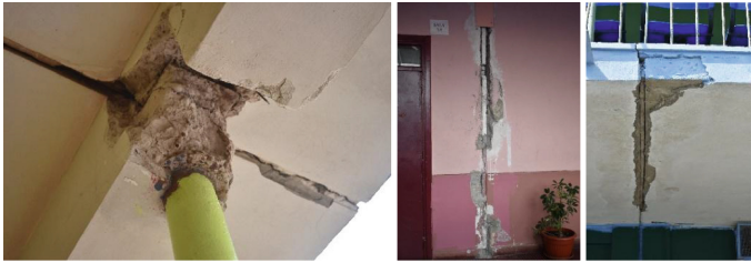
Fig. 3. Faults in expansion joints in all buildings in the sample
