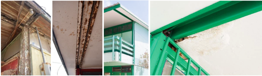
Fig. 5. Corrosive processes in metallic structures with different protection levels (paint).
