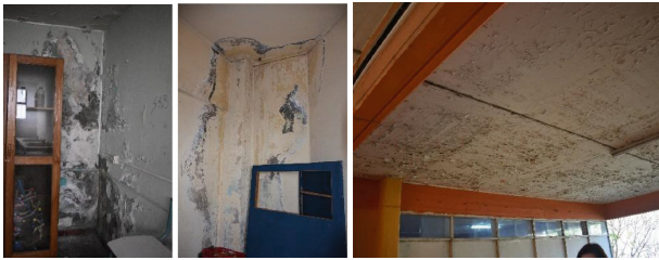
Fig. 4. Stains, efflorescence and peeling paint because of humidity. Absorption by capillarity in retaining walls (Arica) and rainfall leakage (Valparaiso), environmental humidity from morning fog (Antofagasta).
