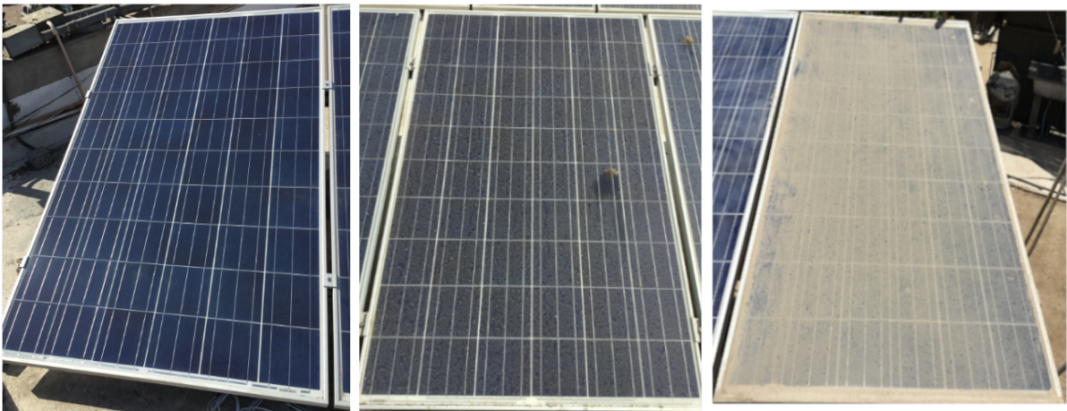
Figure 2.10: Different degrees of soiling deposited on modules surfaces detected by visual inspection.
