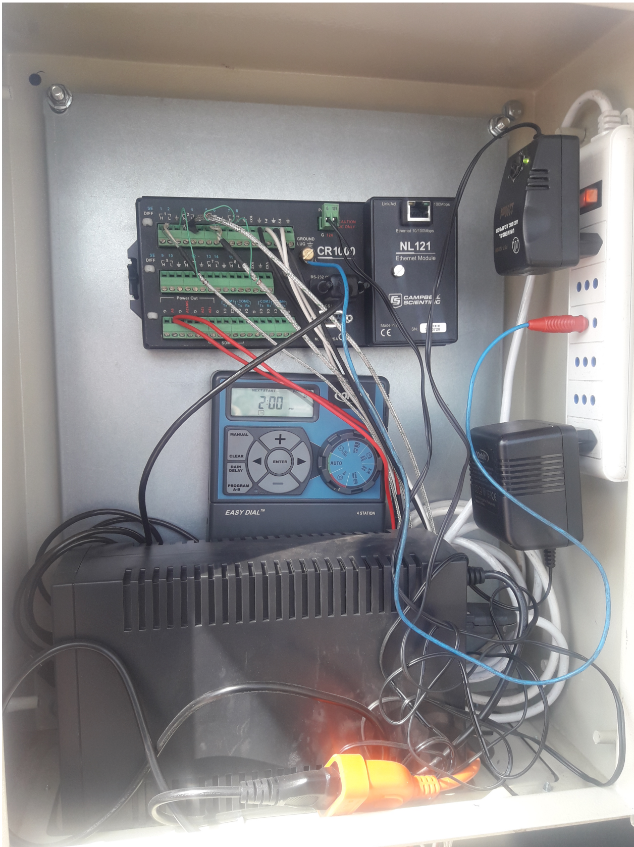
Figure 3.4: DataLogger(above), programmable electric actuator (middle) and UPS (below). Installed inside a safe box
