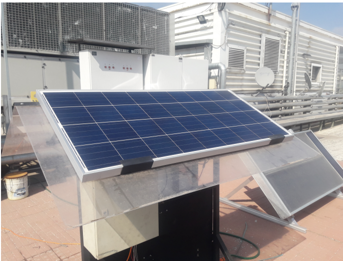
Figure 3.2: PV module installed at a 30 degree tilt, in a setup equivalent to an insulated rack mount
