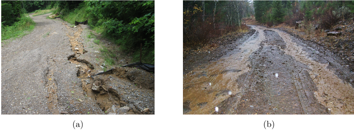
Figure 4.1: Surface Erosion (a) and Surface Runoff (b)
