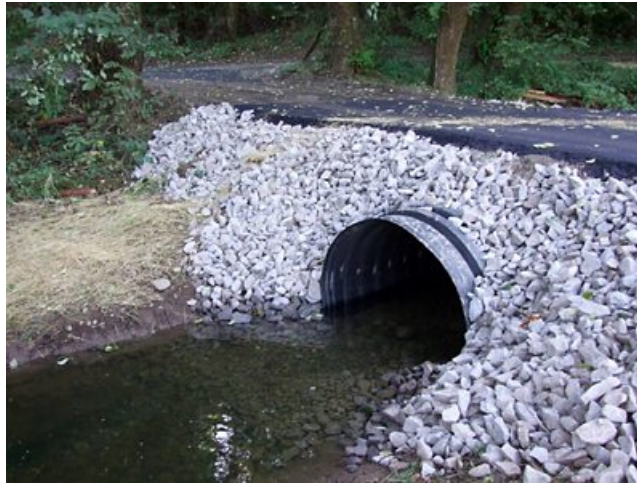
Figure 4.3: Culvert: A tunnel carrying a stream or open drain under a road or railway. They are designed to preserve the channel structure allowing water and fish passage.
