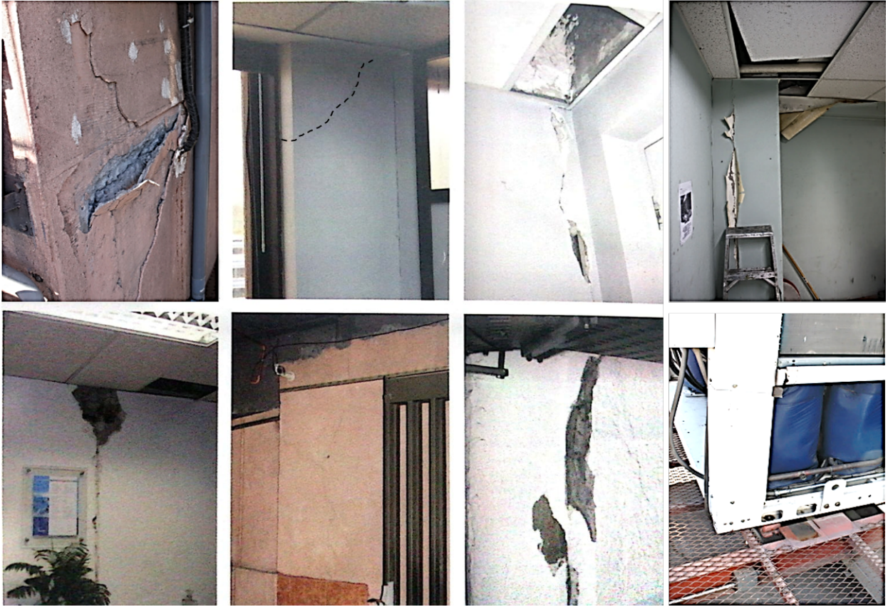
Figure 3.10: Structural and non-structural damage for 27F event in the CChC Building (Photos: Bartolomé & Caroca, 2010 [47]).
