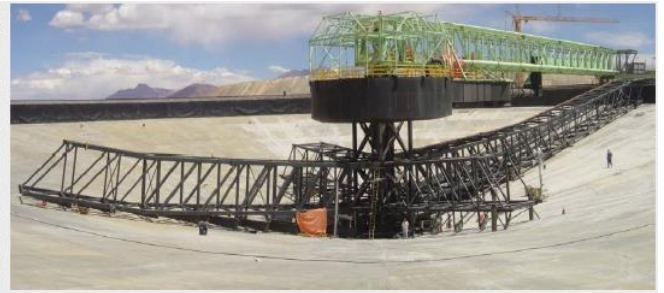
Tailings Thickener, 125m diameter P-DUC® Forced Dilution System Traction Thickener On ground.
