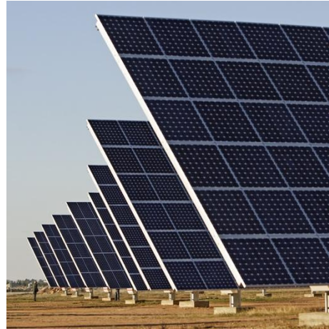
Fig.20; Panel solar normal.
