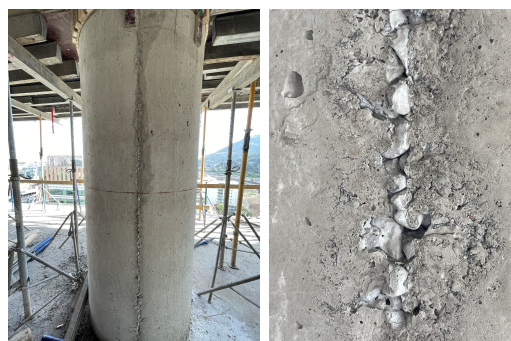
(a) Pilar Defectuoso (b) Defecto
