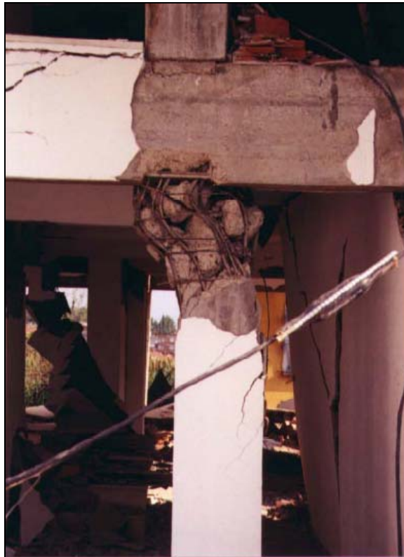
Ilustración extraída de "the august 17, 1999, kocaeli earthequake-damage to structures" (ref. 12)
