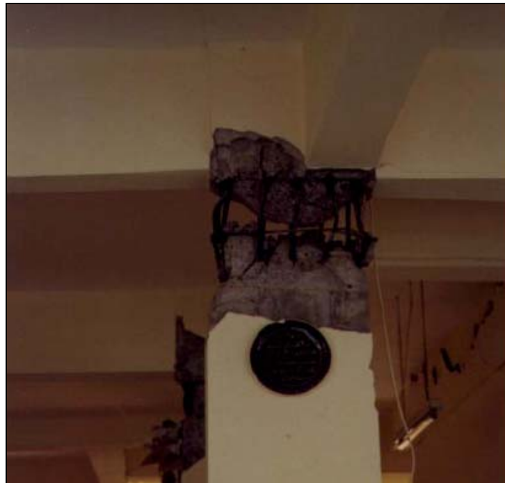
Ilustración extraída de "the august 17, 1999, kocaeli earthequake-damage to structures" (ref. 12)
