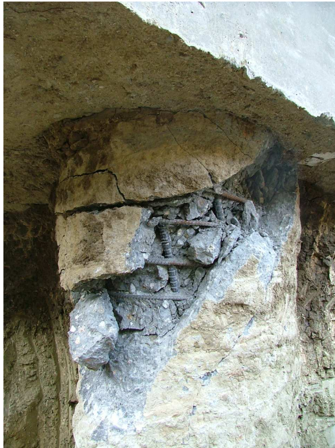
Figure 5.9: Shear cracks observed after excavation. Lemnitzer et al ,2013.
