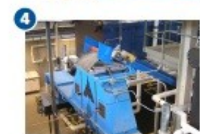
Two traveling augers move the stored woodchips from the bunker onto a conveyor belt that takes them first to the metering bin, where oversized pieces are screened out, before delivering the fuel to the combustor in either of two Messersmith biomass boiler units.
