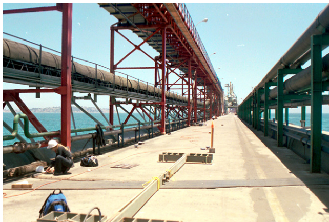
Fig. 3. General view of top deck systems. Note the pipes and frames running in the longitudinal direction that may provide some degree of restraint between adjacent sections.
