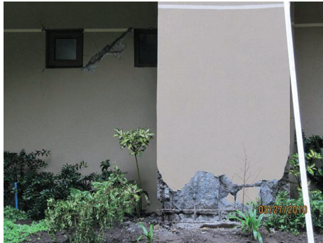
Figure 10. Crushing at exterior wall between lines 4 and 5.
