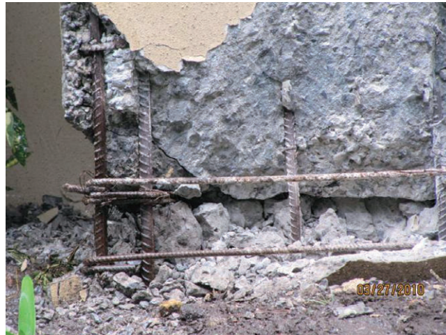
Figure 11. Close up view of concrete crushing and rebar between Lines 4 and 5.
