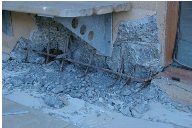
Figure 15. Concrete crushing at edge of 'outrigger wall' along gridline 15.
