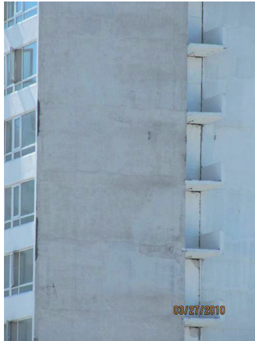
Figure 26. Close view of cracking at extreme edge with repairs made.
