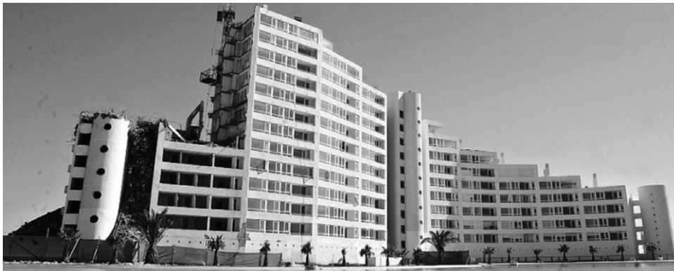
Figure 29. Demolition work caused by damage from earthquake, as of August 2010 (source: http://i857.photobucket.com/albums/ab134/roogenial2/olasim.jpg ).
