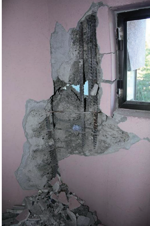
Figure 24. Close-up of interior damage at an edge of the stairwell.
