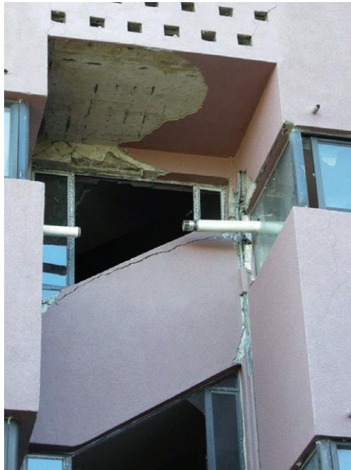
Figure 21. Damage at ends of stairwell.
