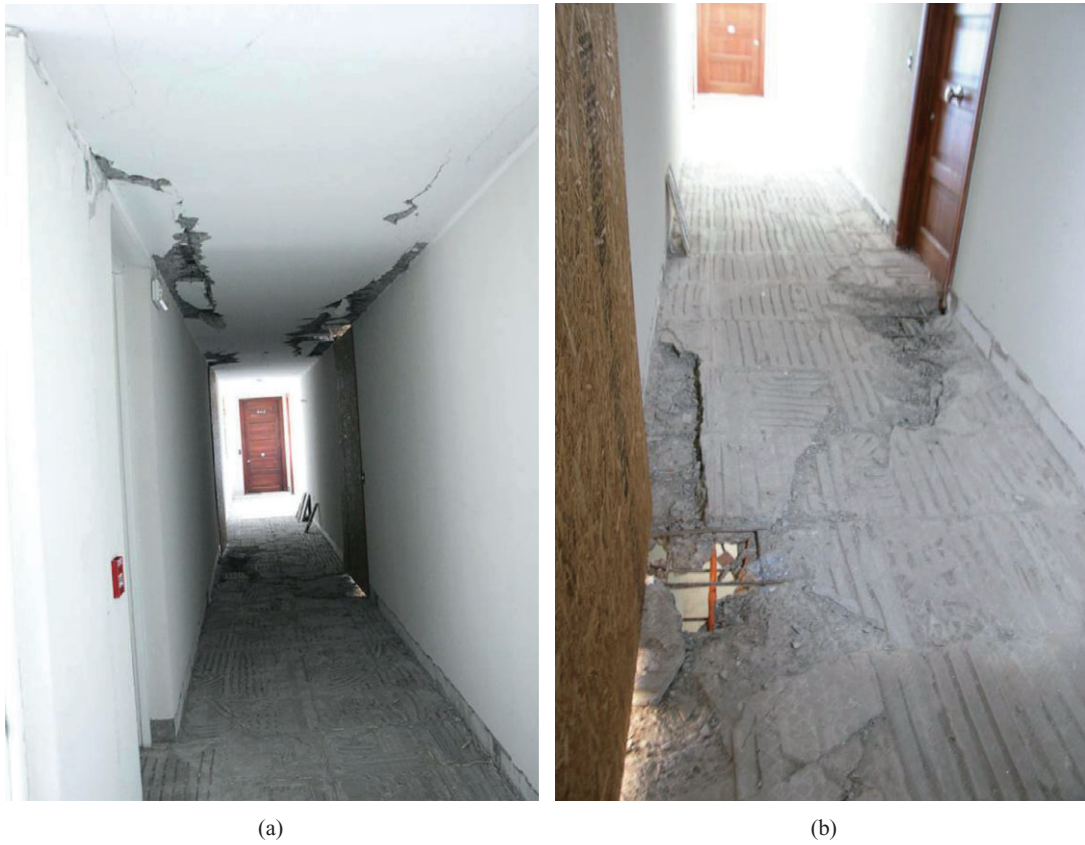
Figure 17. Slab coupling damage.
