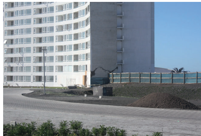
Figure 27. View of damage of end walls after earthquake and before repairs.
