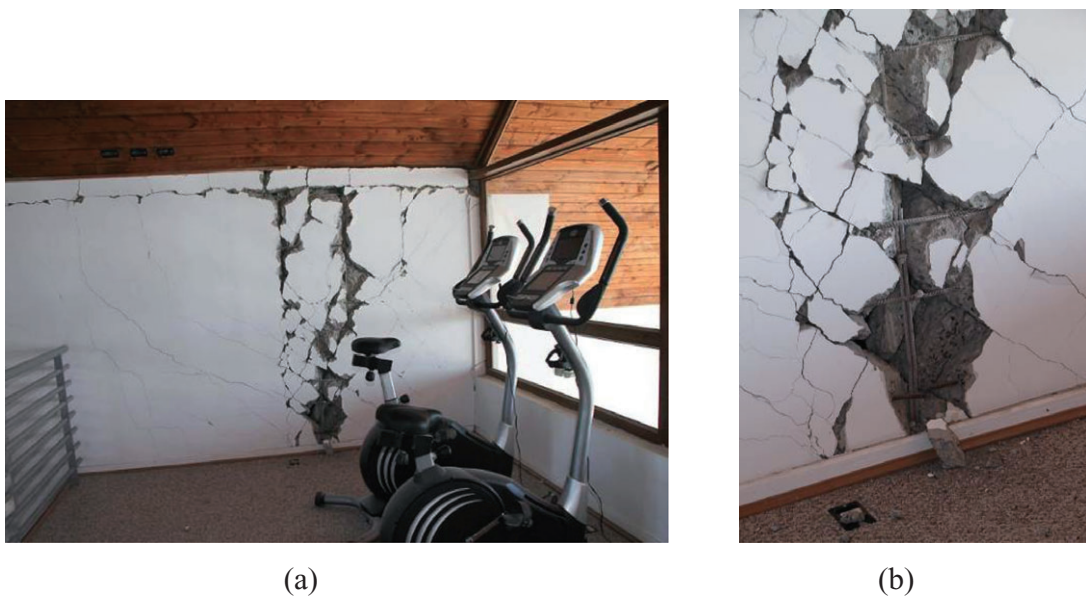
Figure 18. (a) Large cracks at gridline 15; (b) lap splice concrete spalling.
