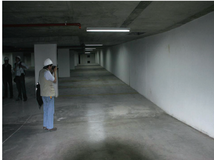
Figure 16. A photo of the Echeverria Izquierdo building at the ninth subterranean floor where no damage was observed to basement walls or floors.
