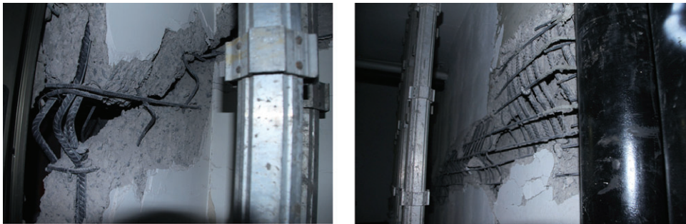
Figure 22. Typical wall damage (note lack of seismic hooks and buckling of main bars).
