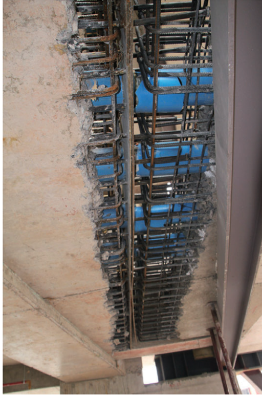
Figure 15. Damage to bridge due to relative movement of the wings.
