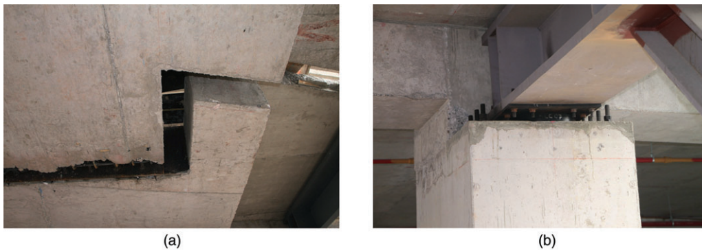
Figure 14. Bridge Details. (a) Separation gap at the bridge-wing junction. (b) Isolation bearing supporting the bridge truss.
