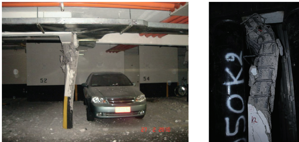
Figure 20. Severe buckling of the walls at the first subterranean floor level.
