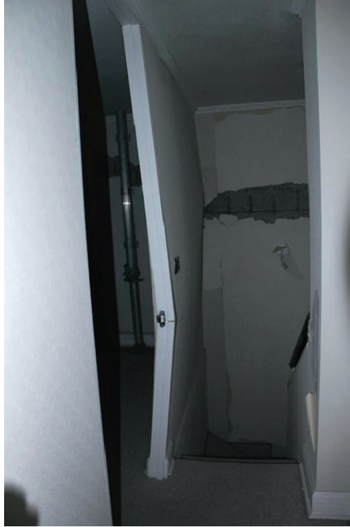
Figure 21. Shortening of floor height causing buckling of non-structural panel.
