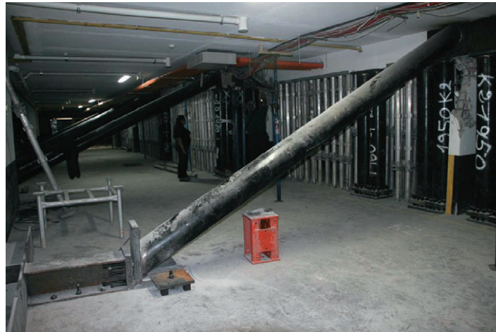
Figure 23. Extensive post-earthquake shoring implemented in the subterranean levels to prevent further leaning of the building to the side.
