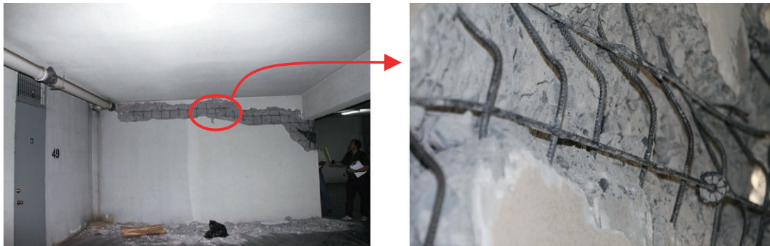
Figure 18. Typical below ground damage at the Central Park building.
