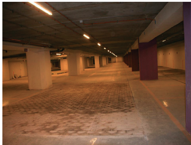
Figure 11. No damage occurred at any of the seven subterranean floors or the basement walls in the Titanium Tower.
