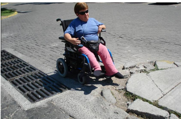
Fig. 1.1. Broken pavements. These compel wheelchair users to use the road risking their lives.
