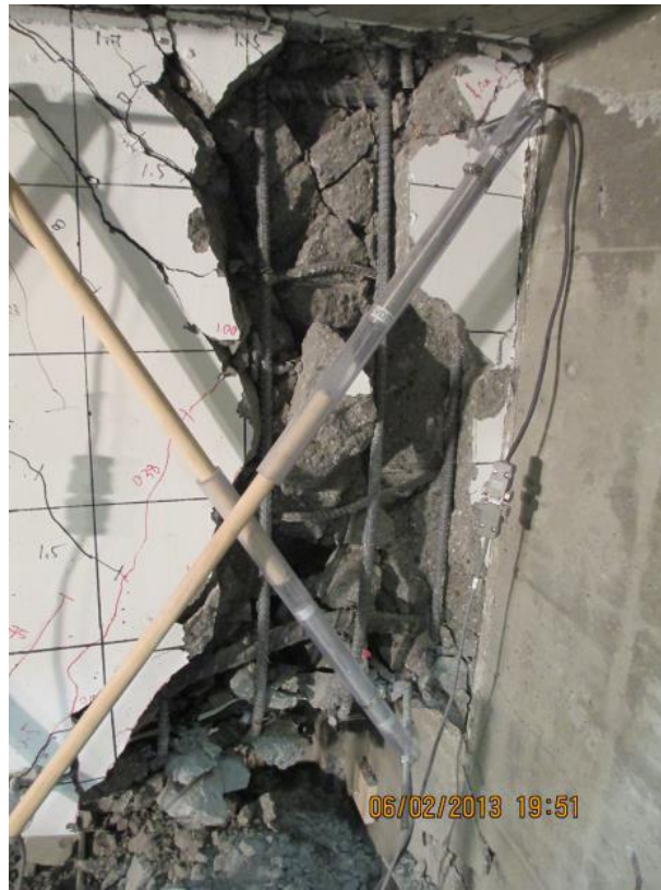
Figure 3.16: Plastic hinge with rebar buckling (Specimen 2), (Lemnitzer et al., 2013).
