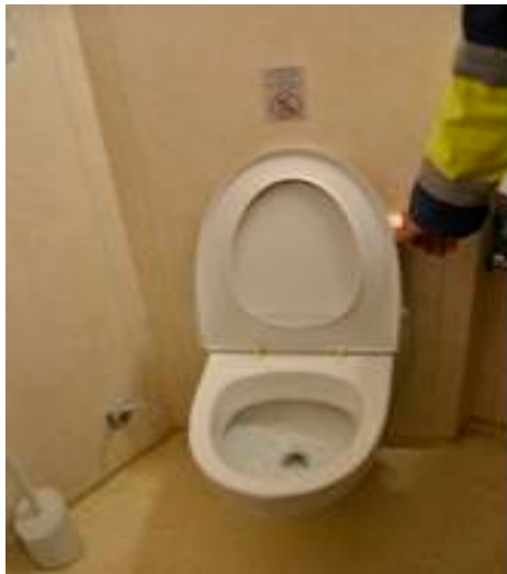
Figure 59. Vacuum toilet (with permission of A. N. Angelakis).
