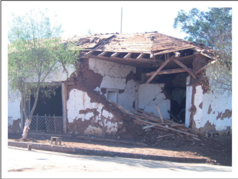
Figure 1. Adobe house in Paredones destroyed by the 2010 earthquake.
