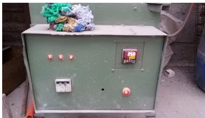
Figura 8 "Panel de control Horno"
