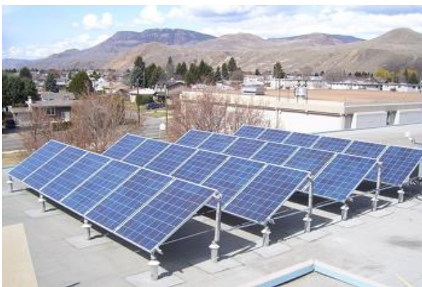
Sistema Fotovoltaico sobre techo plano. Fuente: www.eqmagpro.com/rfs-of-agencies-for-preparation-of-pfrs-for-rooftop-solar-pv-projects-in-india
