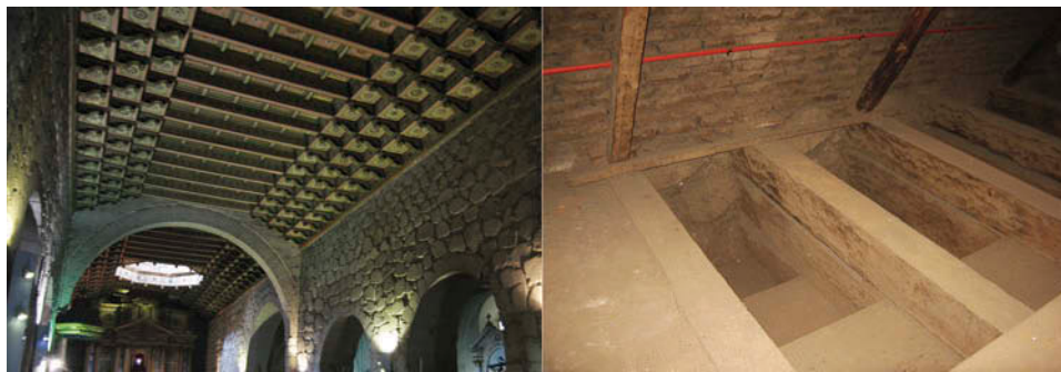
Figure 7. View of the horizontal diaphragm, both from the central nave and from the roof.
