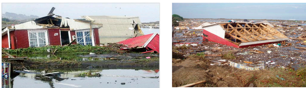
Figure 2. Damage in the San Antonio area caused by the 27 February 2010 tsunami [35].
