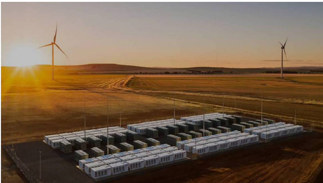
Figura 3.11: Hornsdale Power Reserve en Australia [84].
