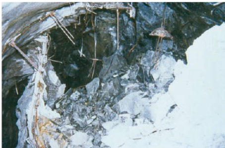
Figure 3—Rockburst damage showing protruding and failed support elements (photograph W.D. Ortlepp)
