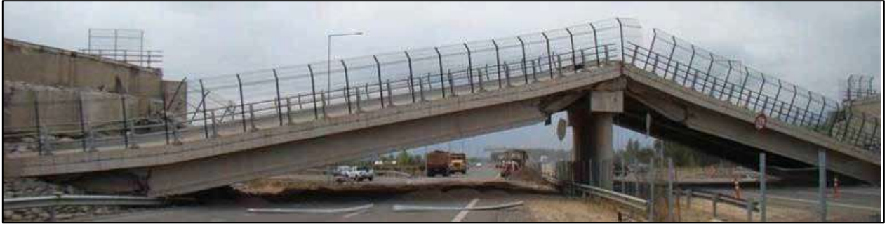
Figura 3: Colapso puente Romeral(Transportation 2011)
