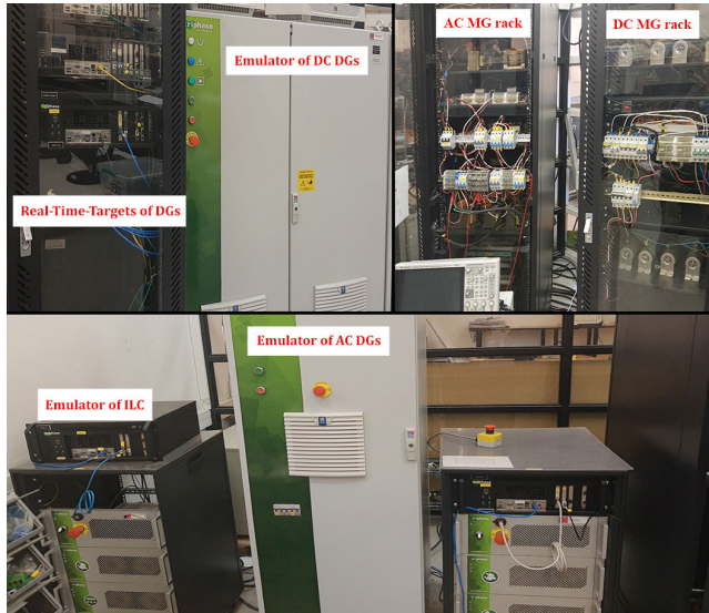
FIGURE 6. Components of experimental testbed hybrid AC/DC MG [33].
