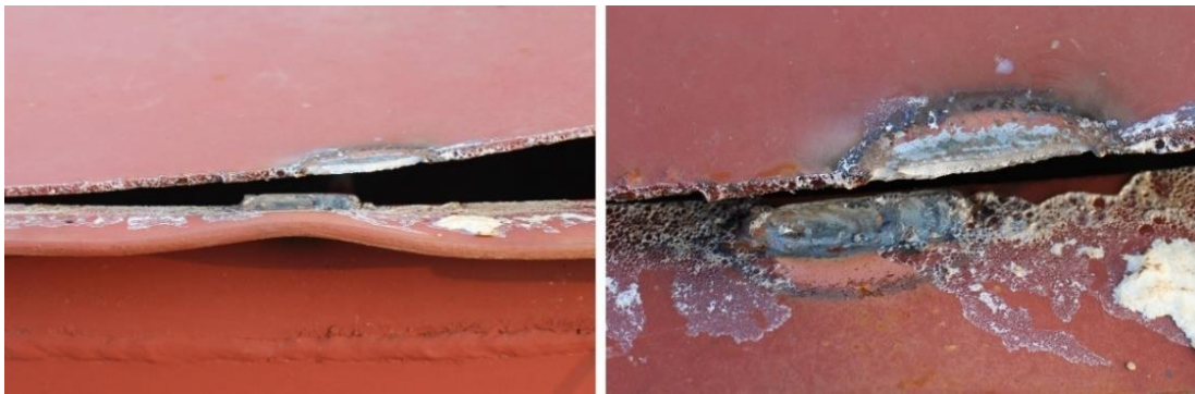
Figure 5: Plasticization of the top ring (left), stitch weld failure during the experiments (right).
